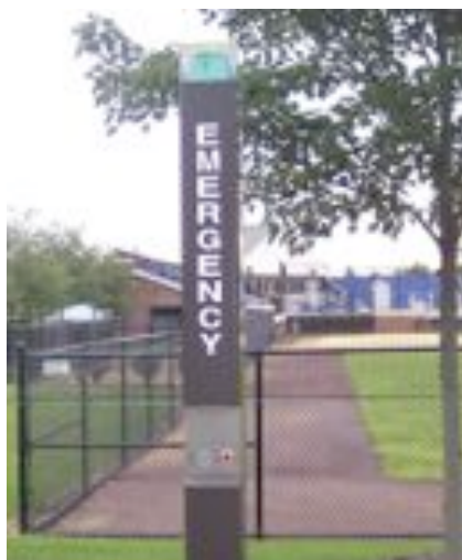
One of the many Blue Emergency Light Telephones on campus.
